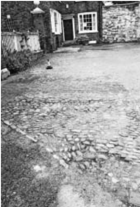
Cobbles in need of repair in Millers Green.
