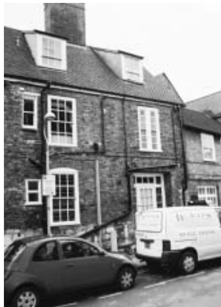
Bad siting of drainpipes, downpipes and exterior wiring and dormers on prominent roof slopes.
