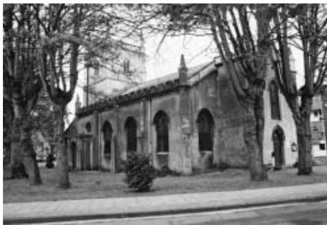
Overshadowed by mature trees and with concrete rendered walls, St Mary de Lode show signs of suffering from the problems of rising damp.
